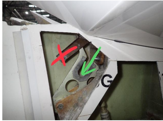
Disconnected elevator control
